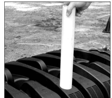
Chamber inspection port.
